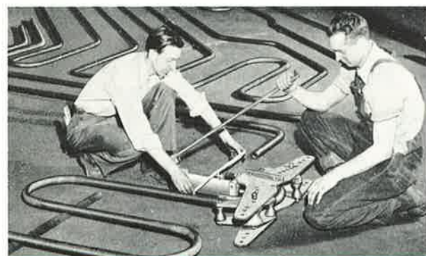
Figure 61: Portable pipe bending equipment makes uniform bends and saves time for The Union National Bank, Pittsburgh, Pa. snow melting installation.
