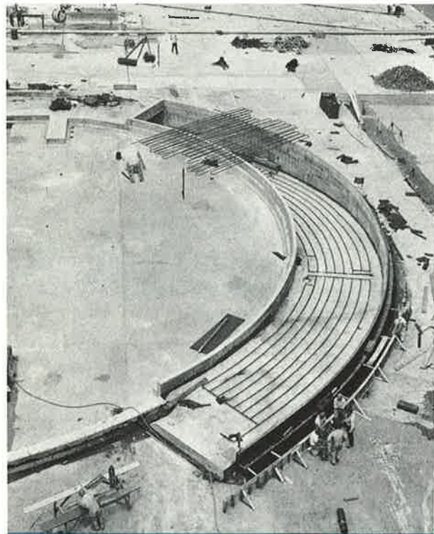
Figure 9 (above): Snow melting system under construction in ramp to parking areas at United Nations Headquarters, New York, Figure 10 (right): Ramp installation at the McCutcheon and Drake Garage, Beckley, W. Va.
