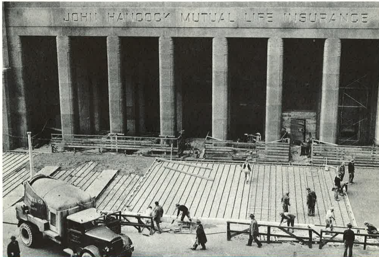
Figure 27: Shown here in the course of construction is one of the largest sidewalk snow melting systems in the world—
